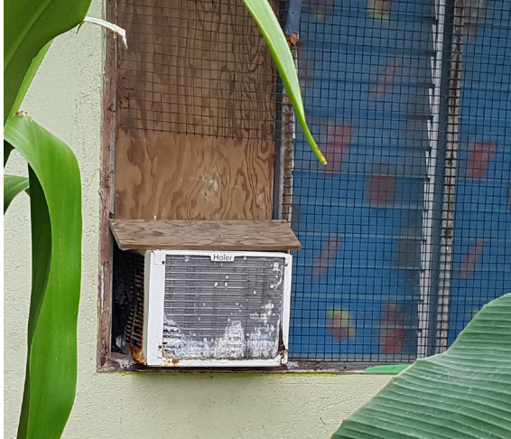
Figure 12: Example of a 'leaky' building envelope and poor efficiency appliance. This window-style air-conditioning unit on Majuro has corroded cooling fins, and is mounted next to louvered window
